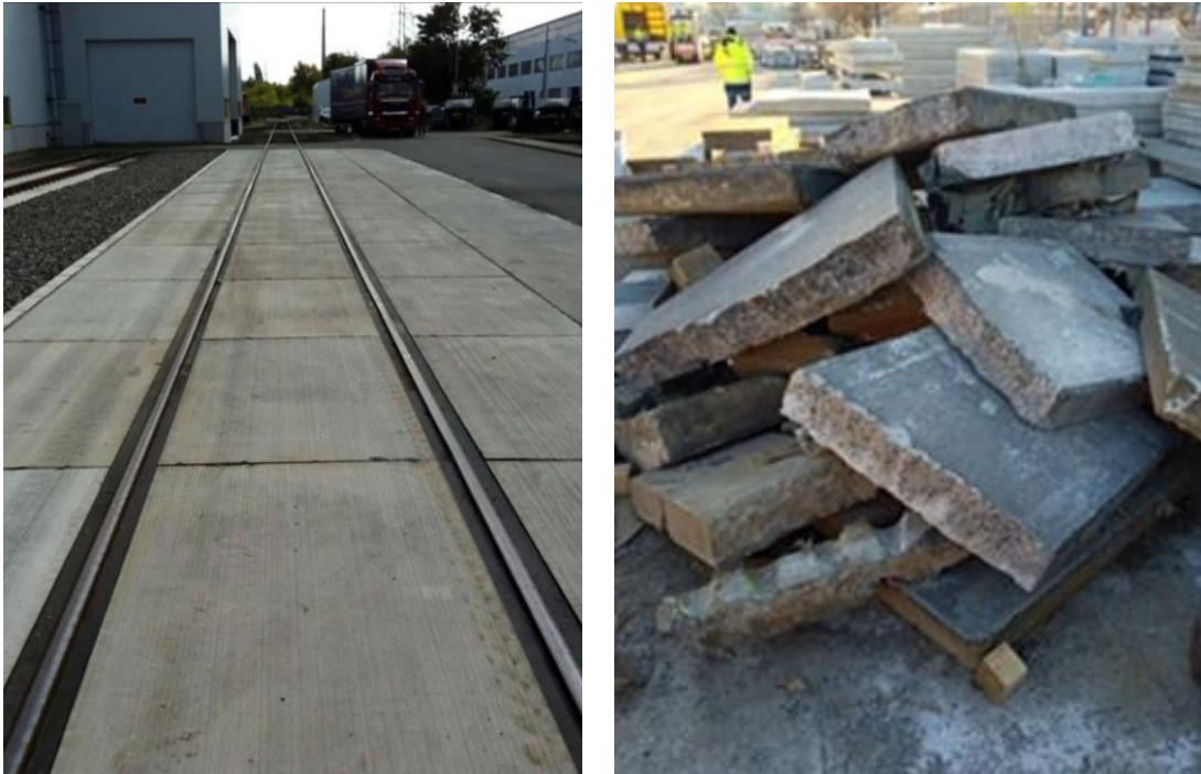
Fig. 21. On the left are panels in the usage phase in the tramway infrastructure, and on the right are the same panels after deconstruction ready for recycling
