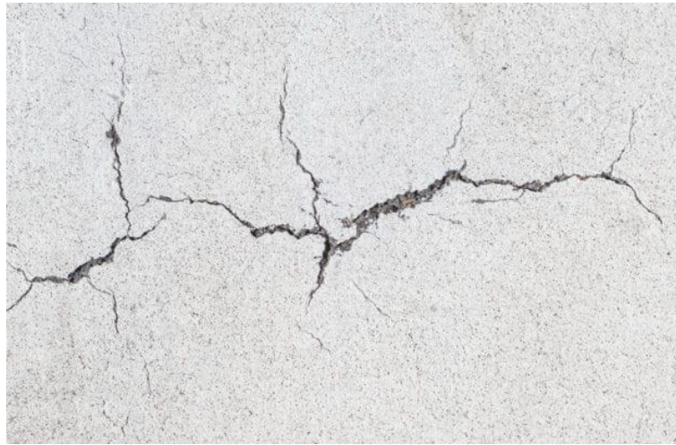
Fig. 7. Cracks on the concrete surface [27]
