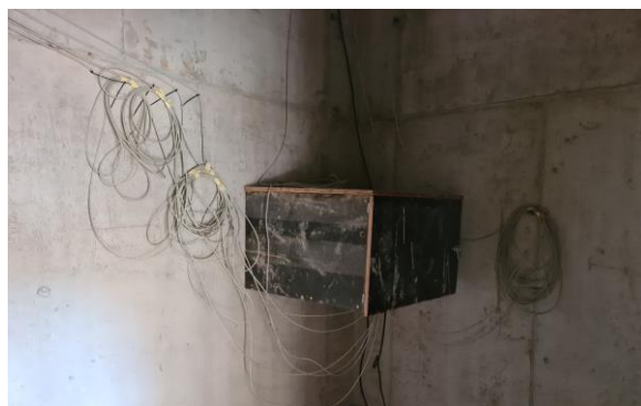
Figure 52. Box containing data acquisition equipment
