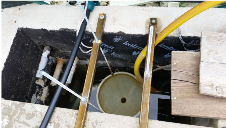
FIGURE A.17: Overflow in downstream reservoir.
