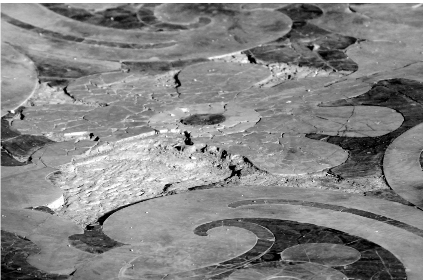
Fig. 5. Pavement of the high altar: some decay phenomena involve the marble slabs
