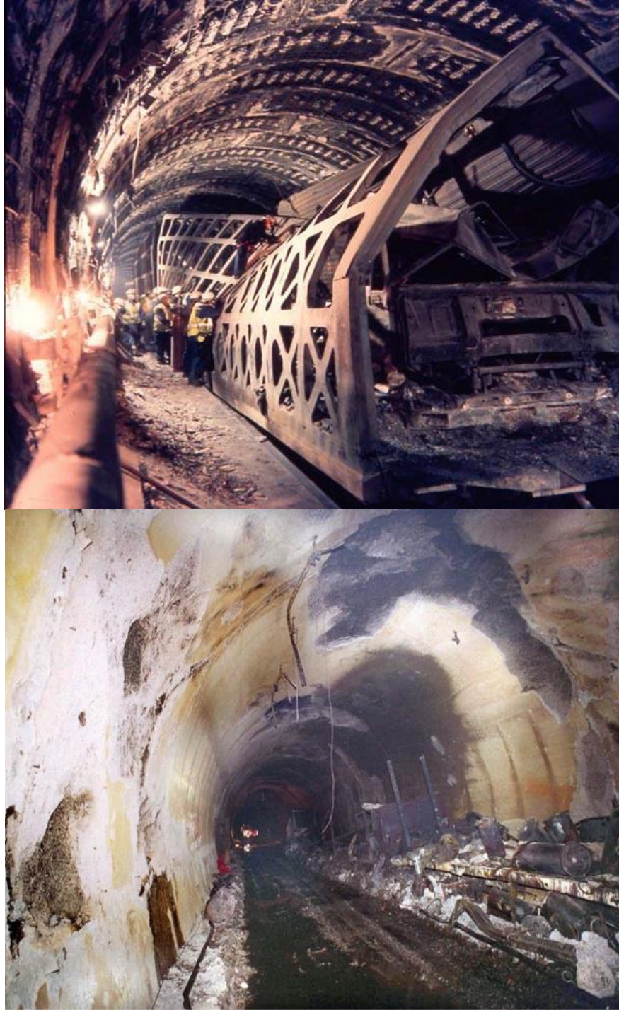
Figure 6: Consequences of explosive cracking of concrete after a fire. (a) Tunnel under the canal after the fire in August 2008. (b) Mont Blanc tunnel after the fire in March 1999 (the image is taken from the source [16]).
