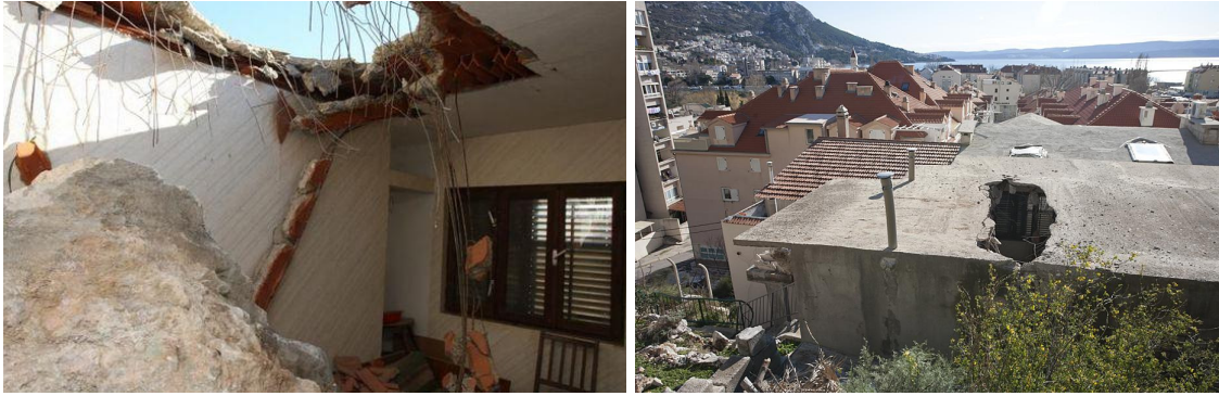
Figure 1.3: Severe damage of houses is caused by rock falls: Omiš, January 2012.
