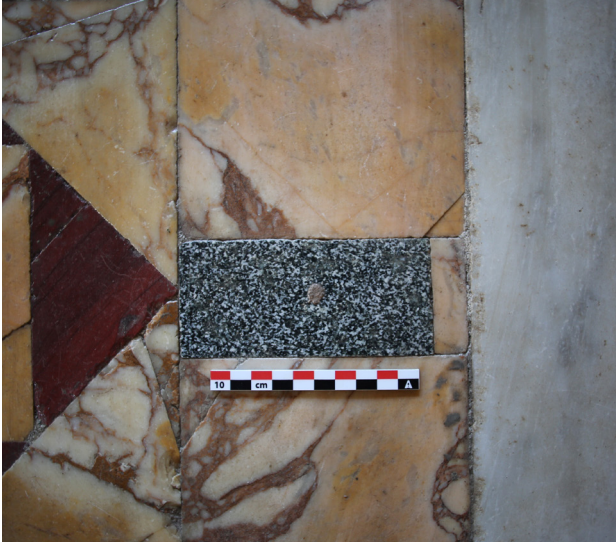
Fig. 17a. Pompeii, House of the Ephebe, Triclinium 17, detail of pavement, granito della sedia di San Lorenzo from Wadi Umm Wikala (photo: S. Barker)
