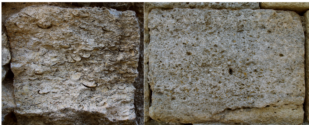
Fig. 10. Blocks of sandy limestone in the pediment of the temple of Jupiter (left) and in the wall of the west entrance zone (right), macroscopic appearance (photo: B. Djurić)
