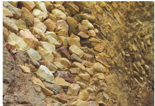
Fig. 11a. Green schist and antique yellow rubble stones used to build the cavea substructions in the Roman theatre (photo: A. Younès)
