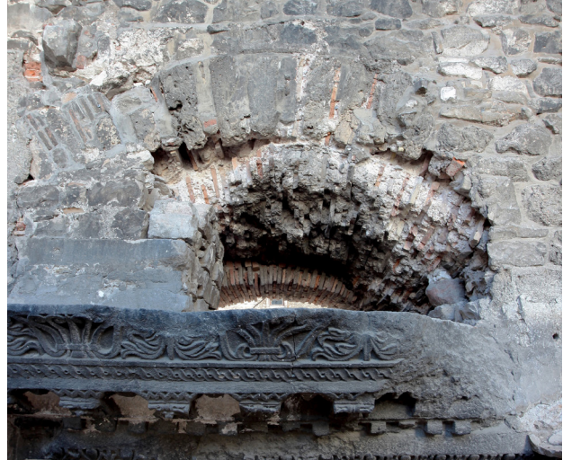
Fig. 4. Peristyle, relieving arch above the portal leading into the Vestibule before restoration (photo: Ž. Bačić)
