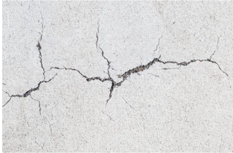
Fig. 7. Cracks on the concrete surface [27]
