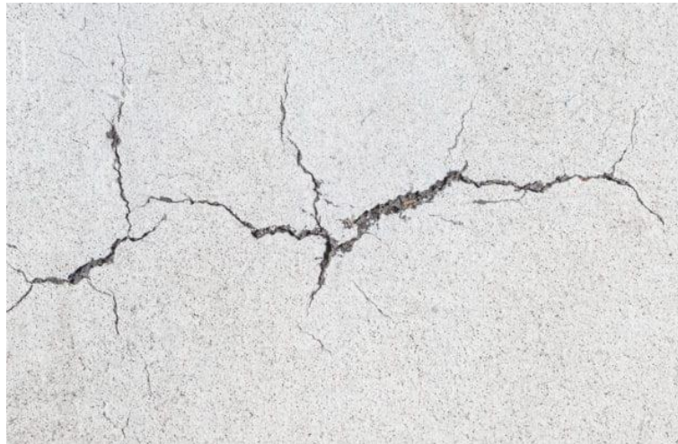
Fig. 7. Cracks on the concrete surface [27]
